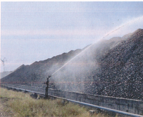
Fig: Dust suppression system in Coal yard
