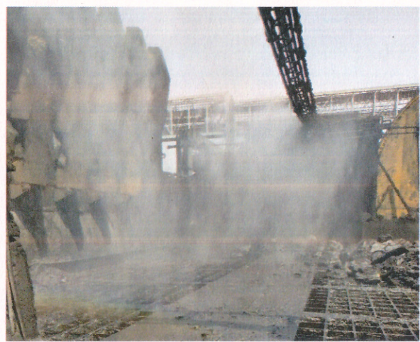
Fig: Dust suppression system in Wagon Tripler
