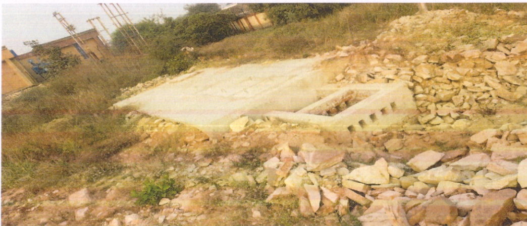
Fig: Rain water harvesting pit: Township
